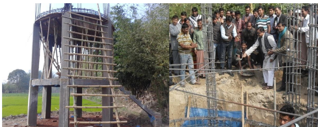
Pipeline water scheme will ensure arsenic-free water 3,000 people of 600 families. (21 December 2014, Howli, Chuadanga)
